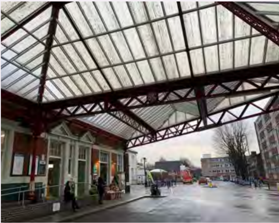
The large glazed canopy with its cast iron columns sits over the station forecourt and entrance and forms part of the listed station buildings
